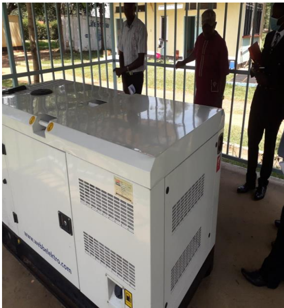
Plate 7: Power backup generator
