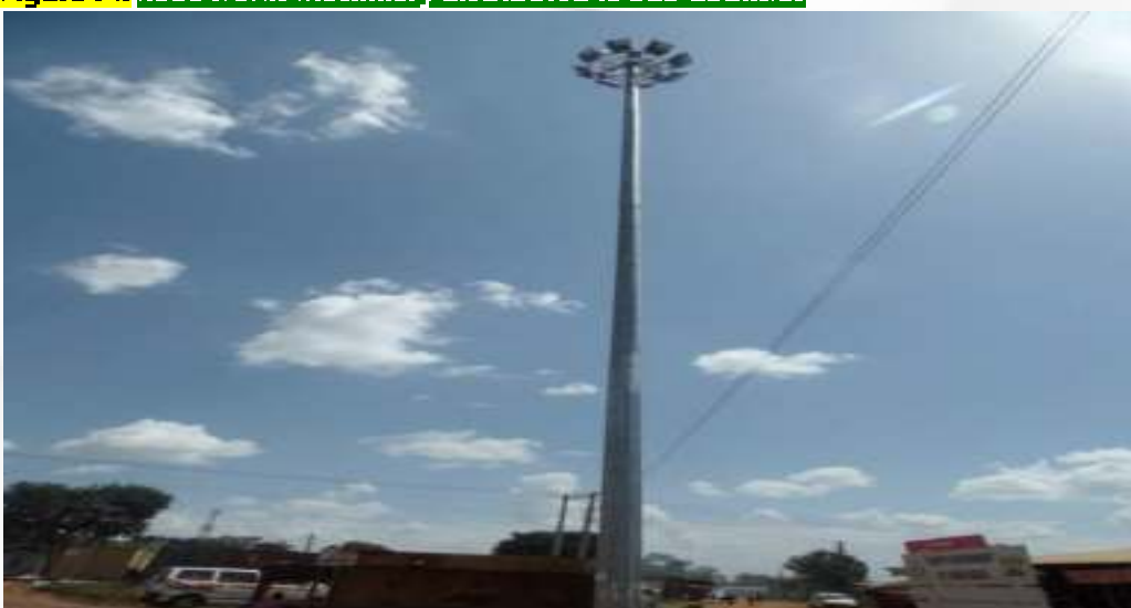
Figure 15: High mast flood light
