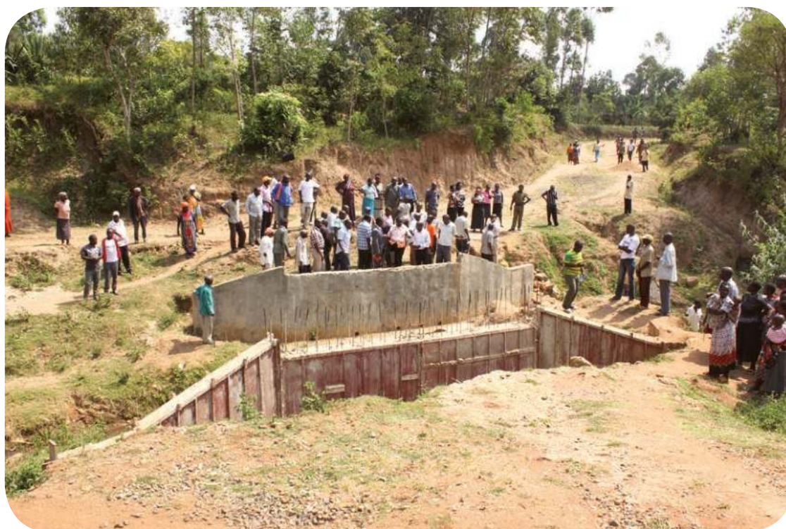
H.E. Governor Wilber Ottichilo and the Transport and Infrastructure team inspecting a stalled bridge in South Maragoli ward
