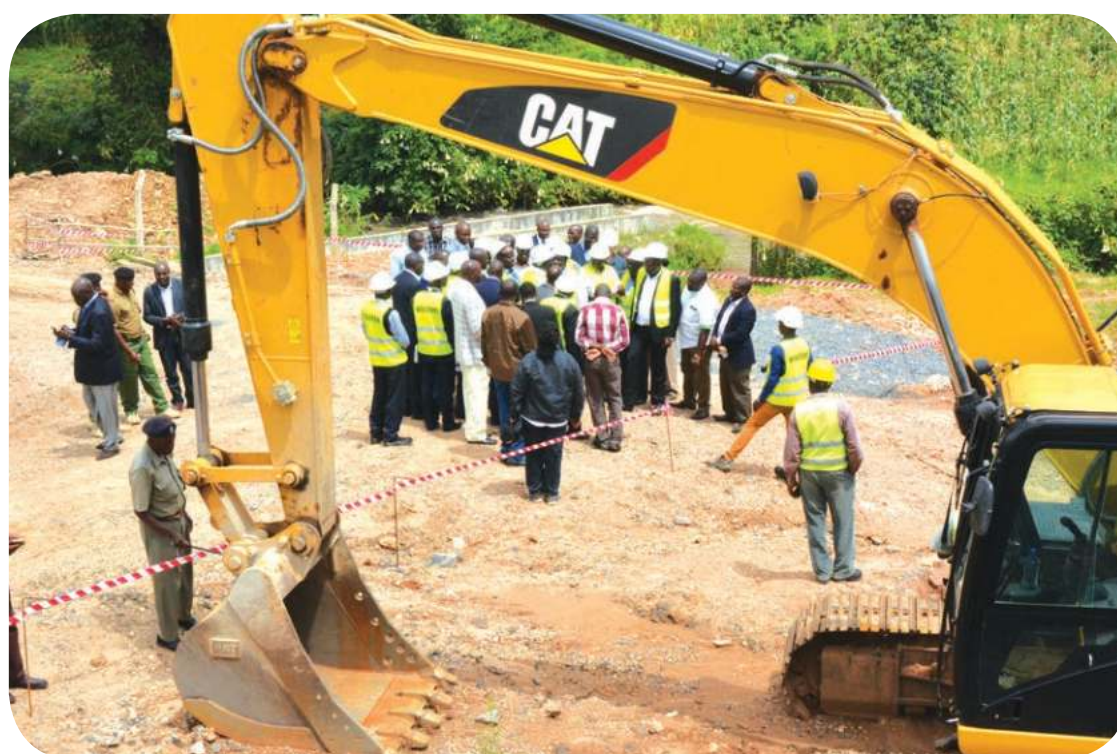
Governor Wilber Ottichilo together with the national CS for water Simon Chelugui inspecting the progress of the KES 1.8 billion, Belgium water project
